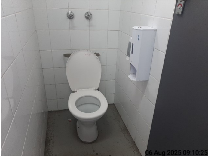
Female toilet -missing tank cover
