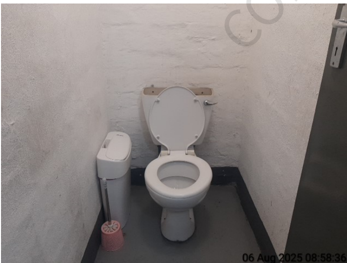
Female toilet-missing tank cover
