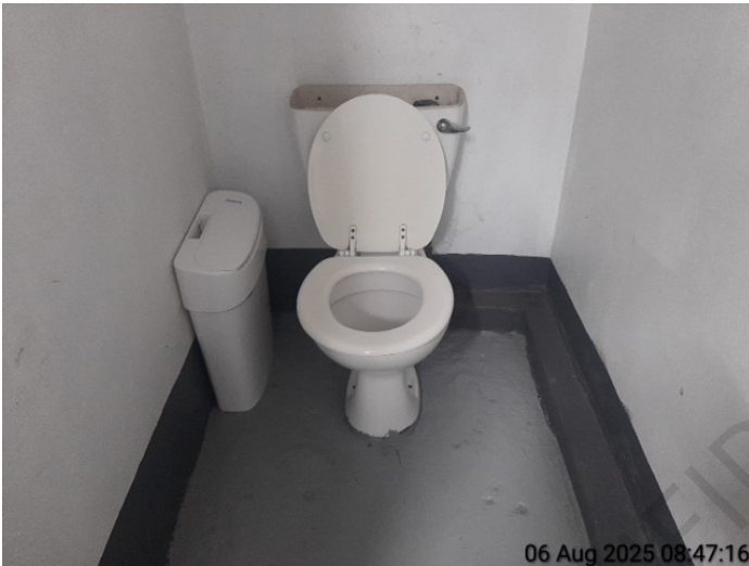
Female toilet-missing tank cover
